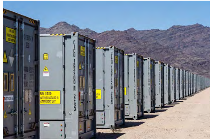
Figure 1: Battery energy storage systems are valuable tools for energy optimization
